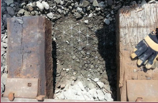
IMAGE A: TriAx TX190L Geogrid was in good condition with no damage observed while continuing to support ballast near the surface.
