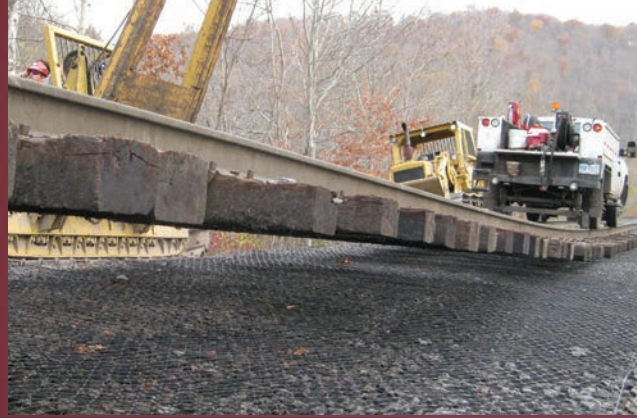
IMAGE D: Existing track can be jacked up so that new geogrid and ballast can be added.
