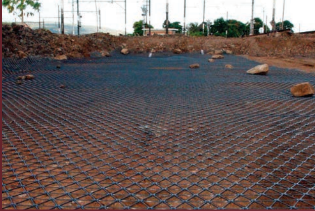
IMAGE C: To stabilize the sub-ballast under a new rail line, geogrids are simply rolled out directly on top of the prepared subgrade.
