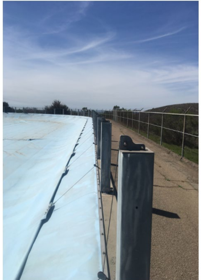
Figure 7. Mechanical Tensioning Tower System on Upper Valley
