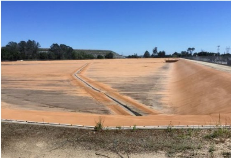
Figure 4. Hinkle Reservoir, 37-Year-Old CSPE Floating Cover Picture 2017
