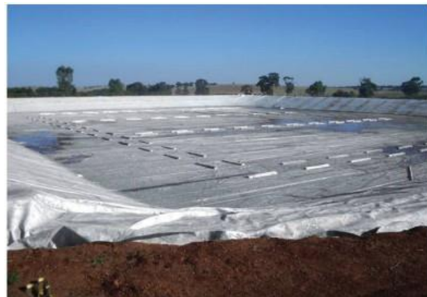
Figure 4. Installed 30 mil (0.75mm) defined sump floating cover in South Australia (Photo courtesy of Fabtech)
