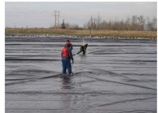
Figure 2. Prototype 30 mil (0.75 mm) cover with field technicians on surface installing weighted sump
