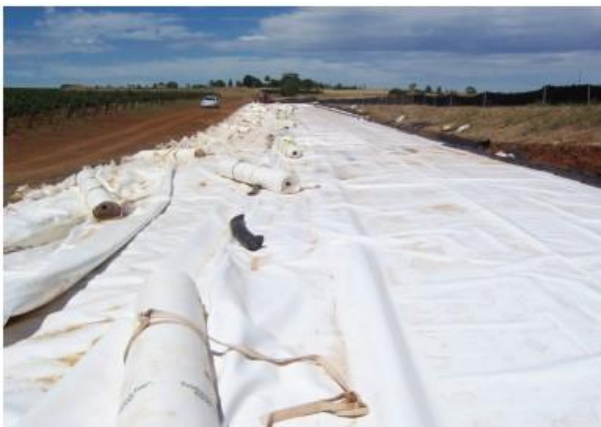
Figure 3. Laydown area for fabrication of 30 mil (0.75 mm) panels in South Australia (Photo courtesy of Fabtech)
